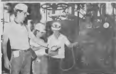
William Smith of Exxon's Research Environmental Health Control along with Rusette Arends and Simon Geerman of Lago's Safety Section are checking for hydrocarbon gasses at a leaking pump, during the two-week annual Environmental Health Control.
